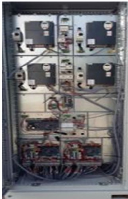
Fan drives + Pump drives + electronic boards
