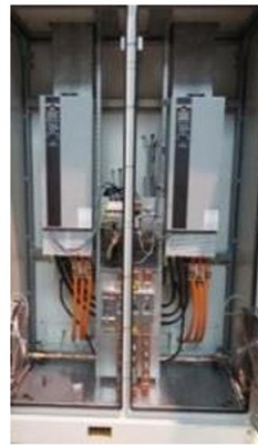
Compressor drives + main power connection
